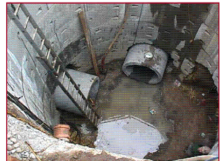
Large Diameter Sewer Outfall through Balbriggan Town Centre, including extensive thrust boring
